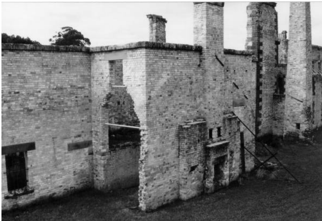
Bakehouse Wall - Additional support required to wall
