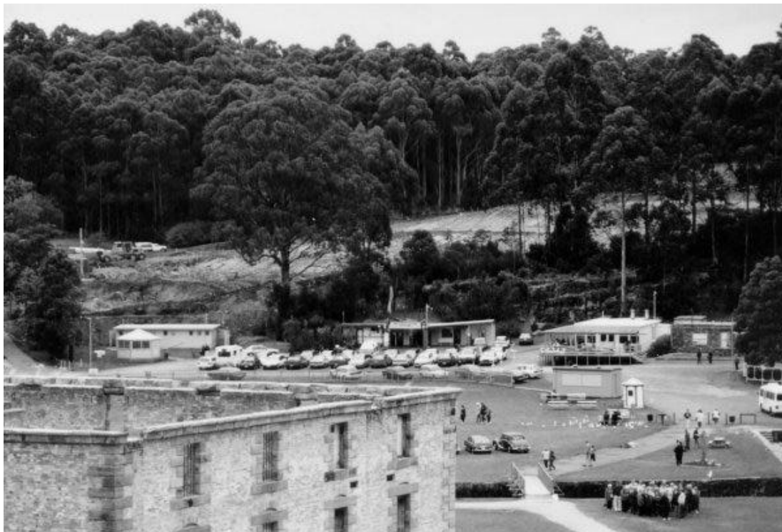
Excavations for the Visitor Centre and Car Park as viewed from behind the Penitentiary.
