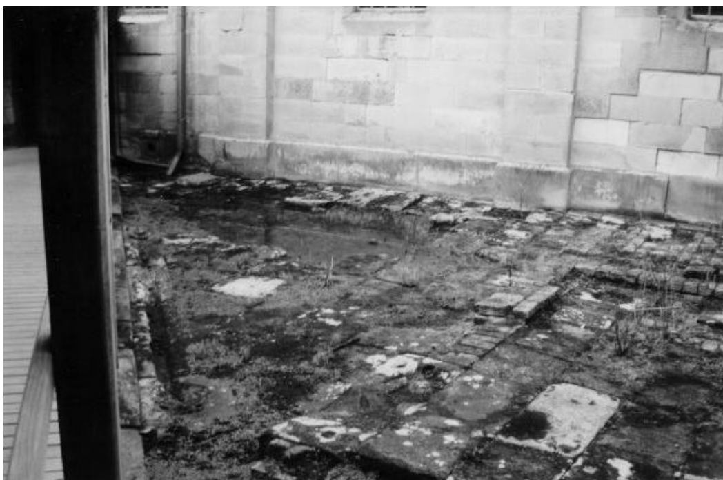
Model Prison - Exercise Yard - Weed infestation and lack of adequate drainage
