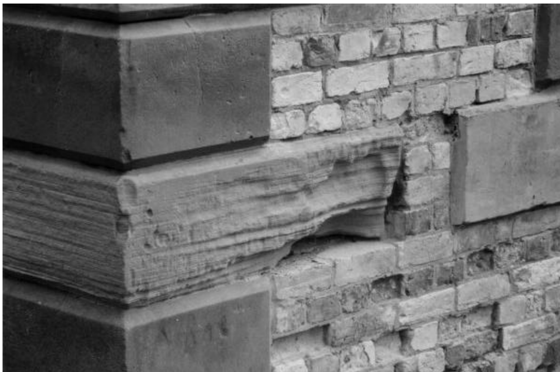
Penitentiary - Sandstone and brick erosion
