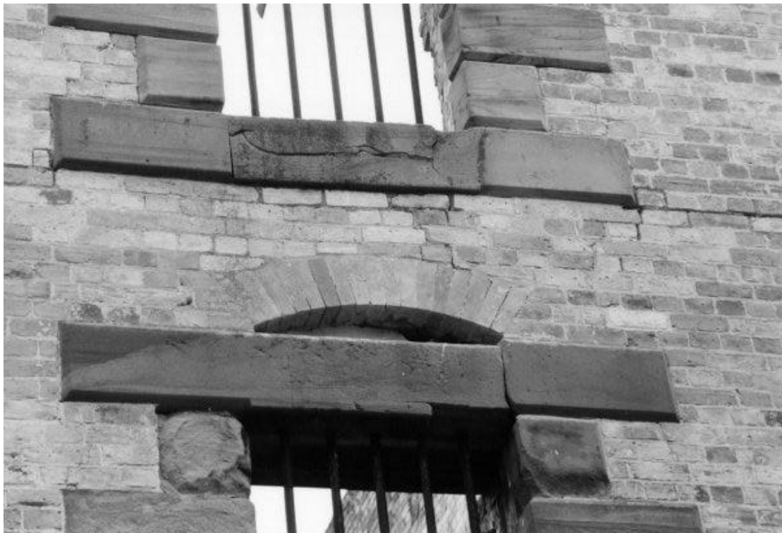
Penitentiary - Broken sill and lintel
