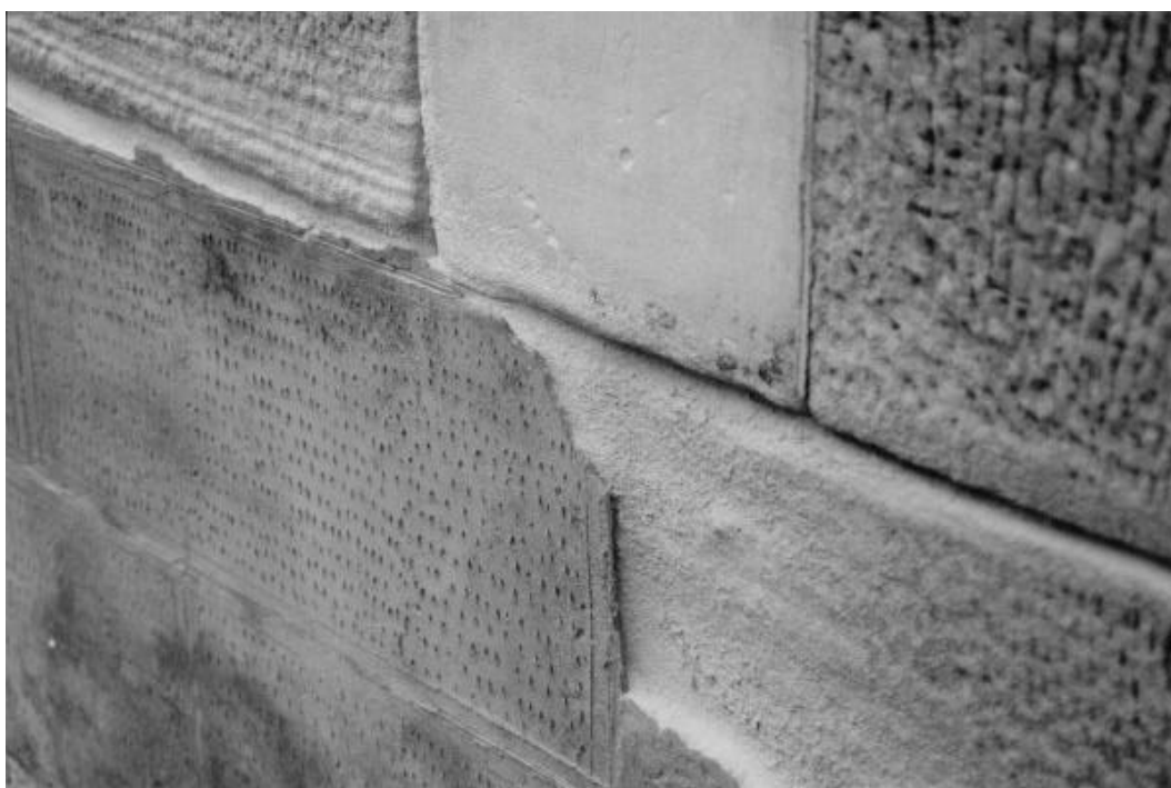
Model Prison - Sandstone erosion behind a previous cement render repair
